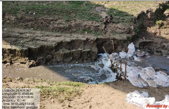
Inadequate tapping of Drain for Treatment Through Geo-Tube
