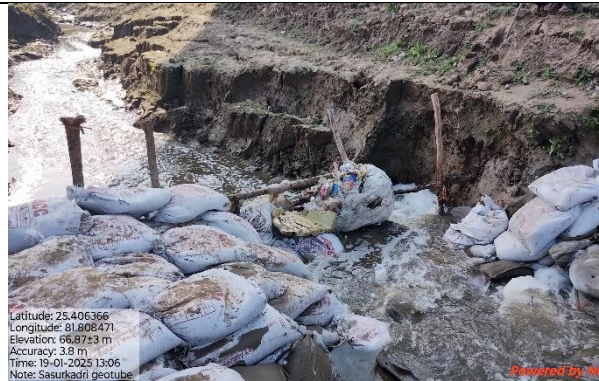
Bypass through Broken Tapping
