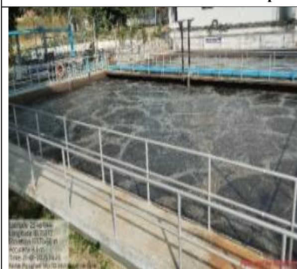
Ponghat STP (Aeration Tank)
