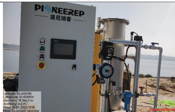
Not working Ozonator
