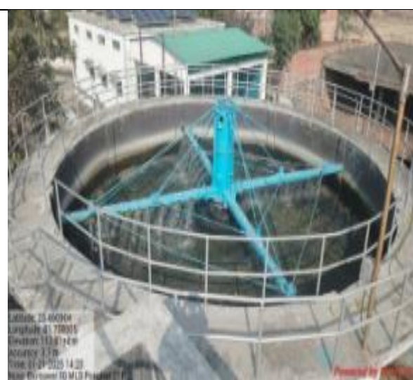
Ponghat STP (Bio-tower)
